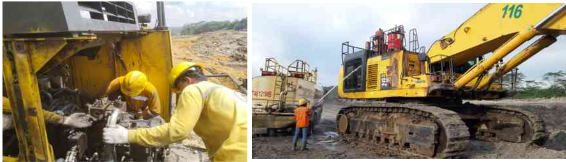
Figure 4.12 Daily check from mechanic and finding in PC1250 Hydraulic System
