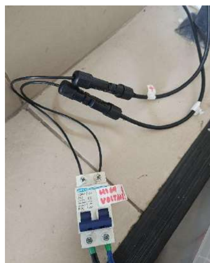
Figure 3.21: Cable Connected to MCB
