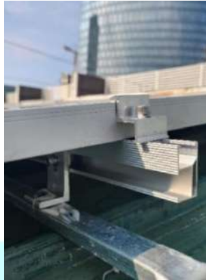
Figure 3.2: Solar mounting system on rooftop
