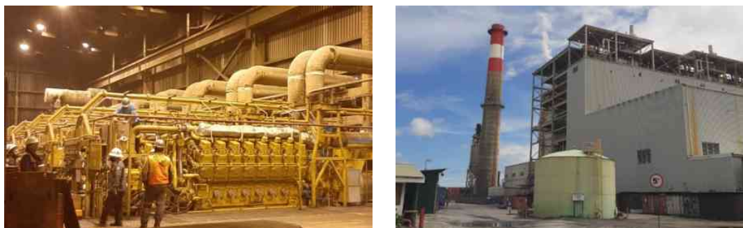
Figure 1.3 (a) Diesel Power Plant (Highland) (b) Steam Power Plant (Lowland)
